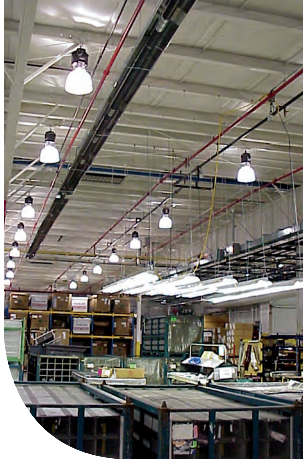
Workstations heated with infrared heaters.
