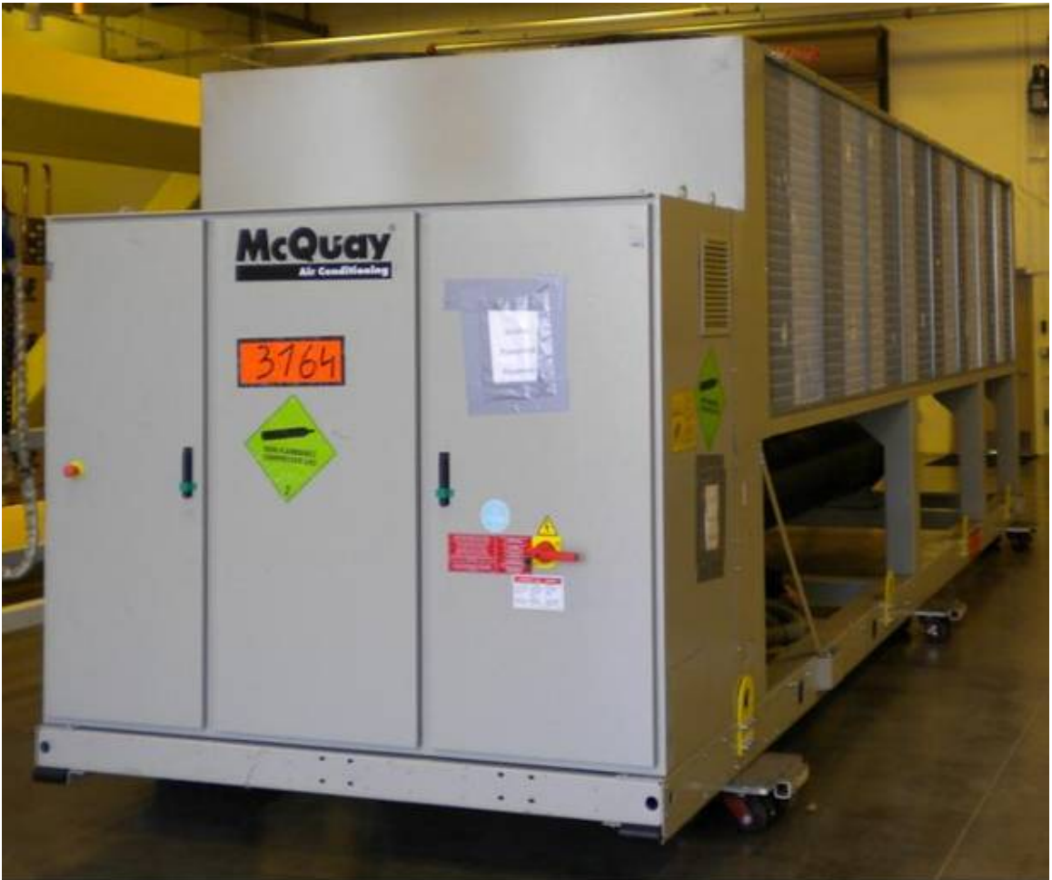
Figure 1. Photo of the Tested Air-Cooled Chiller
