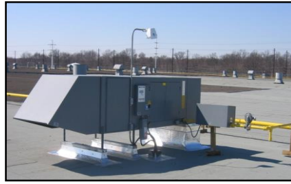
Roof Top Installation
