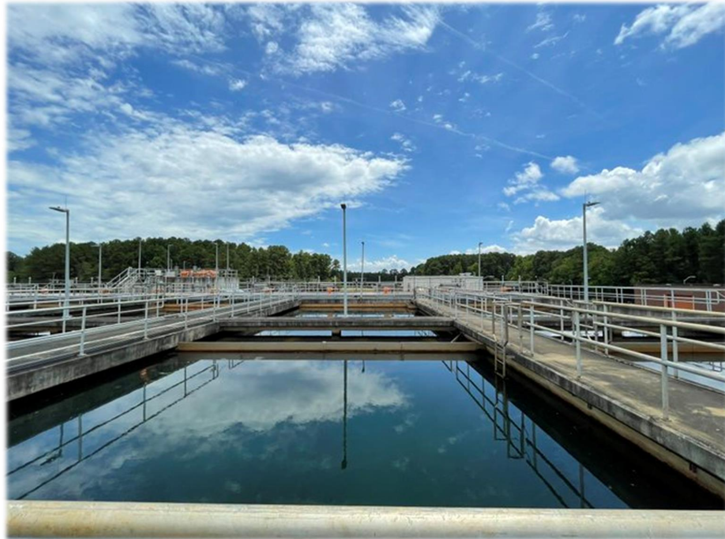
Fayetteville PWC P.O. Hoffer Water Treatment Facility
