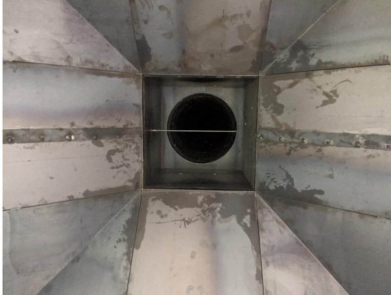
Figure 12 – Top of exhaust hood showing the acid gas probe
